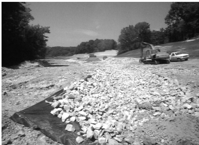
Figure 5. Spreading of 60 cm of FGD by-product on the regarded pile surface (top); construction of diversion channel using a geotextile liner and limestone (bottom).
