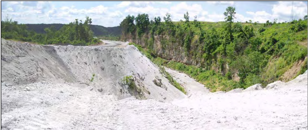
Figure 30 – Starting at one end of the cut, FGD material is placed to fill the old pit and cover the highwall.
