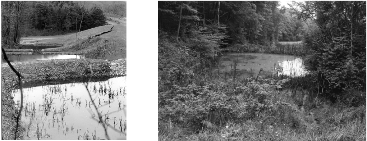
Figure 6. The lined passive treatment system (SAPS) treated the mine discharge at the pile head and discharged the treated water into the diversion channel. In 2006, the system continues to require maintenance.
