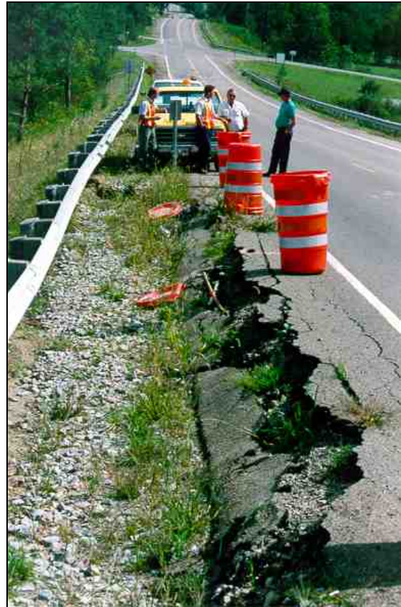
Figure 32 – Existing damage to SR 541 after attempted repairs.
