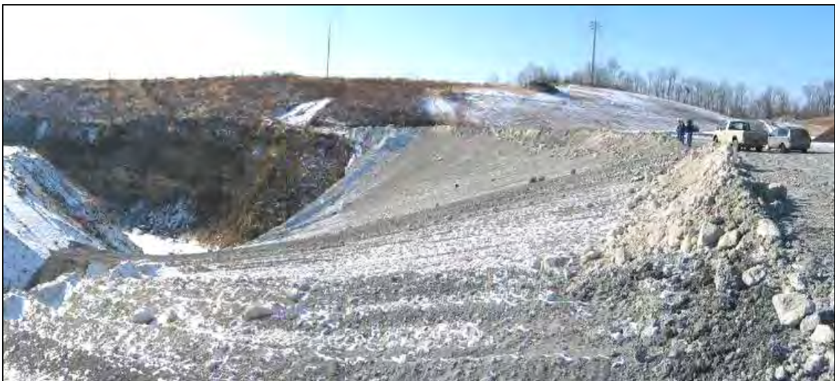
Figure 28 – FGD material placed in one end of the old pit and highwall.
