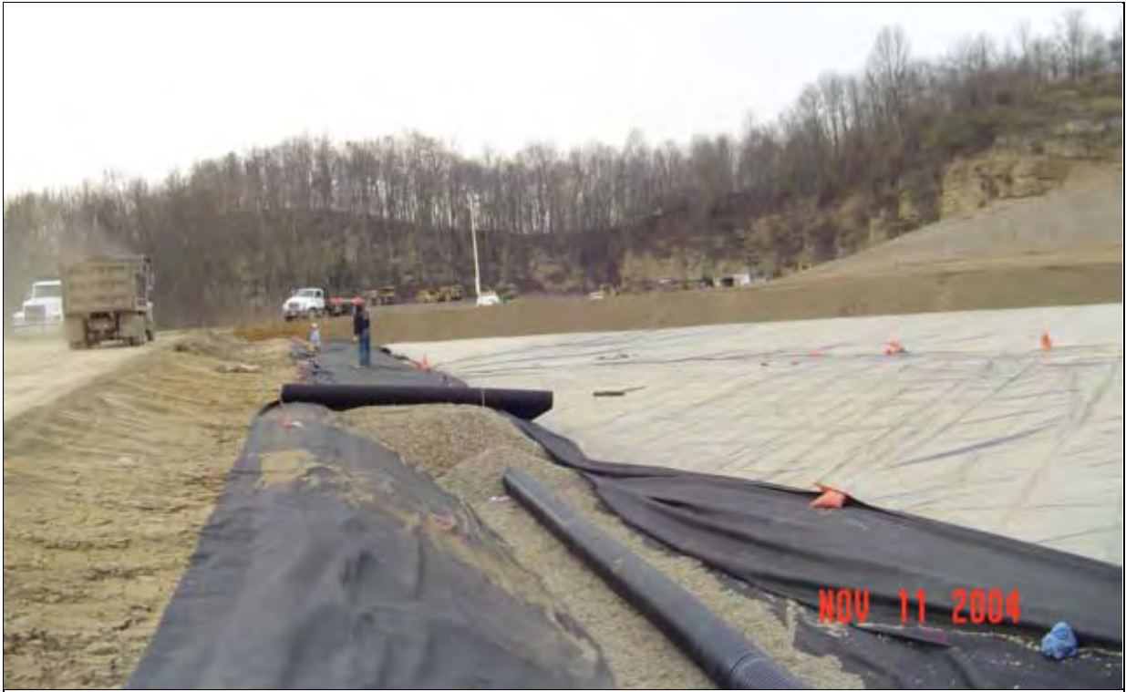
Figure 18 – Leachate Collection Piping, Phase A Area.
