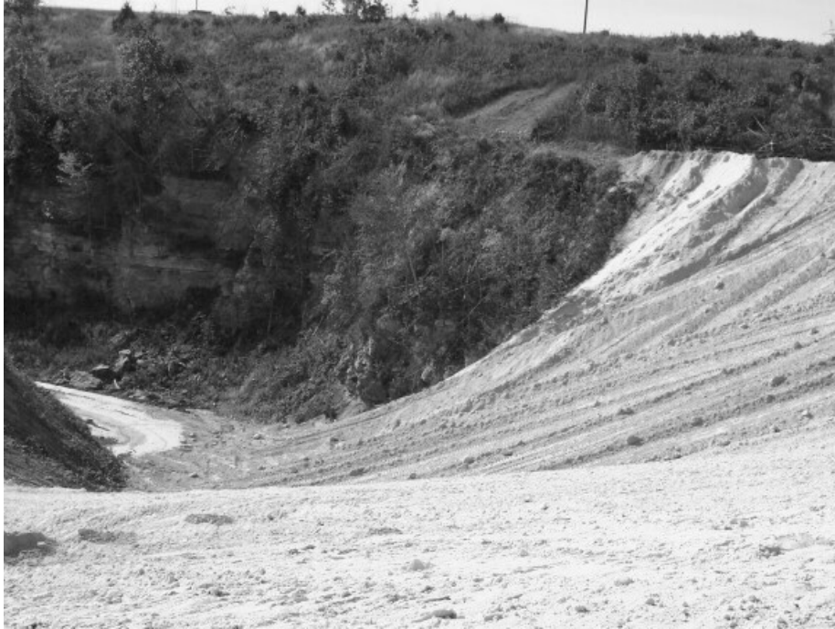
Figure 7. Photograph of abandoned mine site being backfilled and reclaimed using FGD residue.
